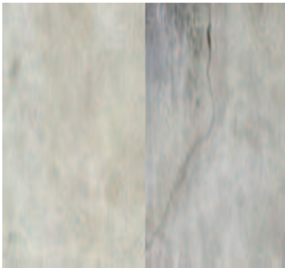
(a) Urban wall (b) Urban wall cracked Fig. 1. Walls in real world environment observed by system using camera.
