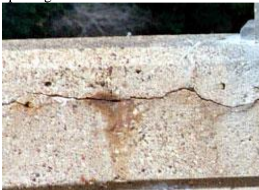
Fig 1.2 Cracking of concrete
