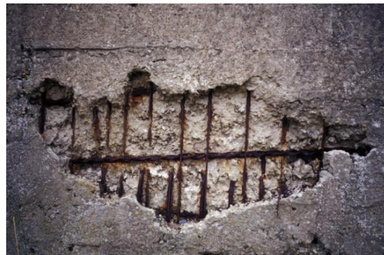
Fig 1.3 Spalling of concrete
